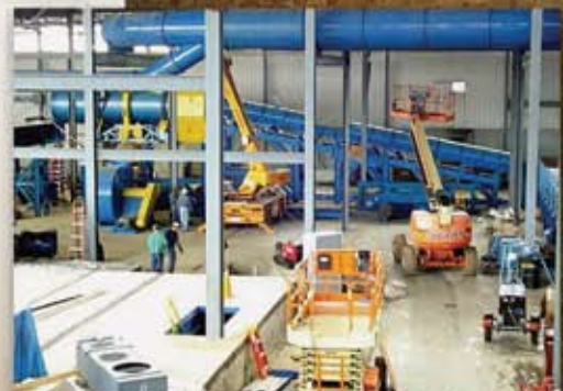
Oct 10 – Molding and casting processing equipment installed.
