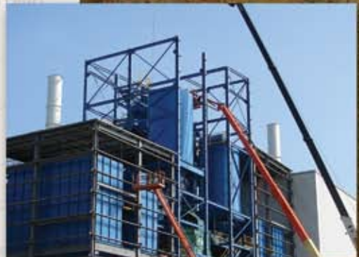
Sept 24 – Last of sand tower equipment installed, coordinated with installation of building siding.
